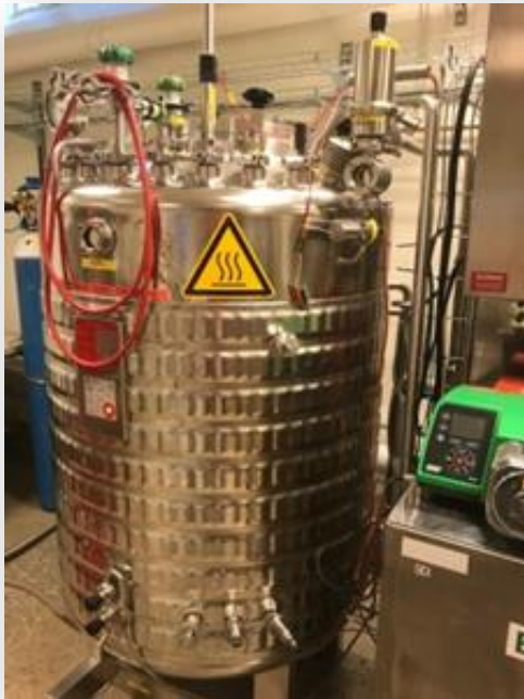
The fermentation reactor of Pilot Line 2
