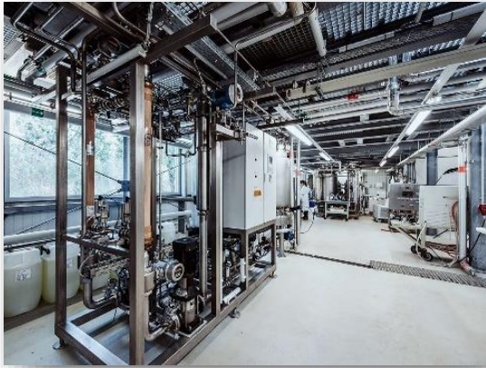
Facilities of Pilot Line 7
